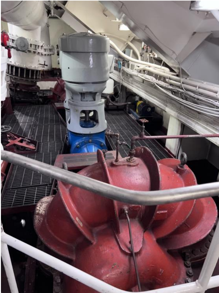
Manifold Ballast System
